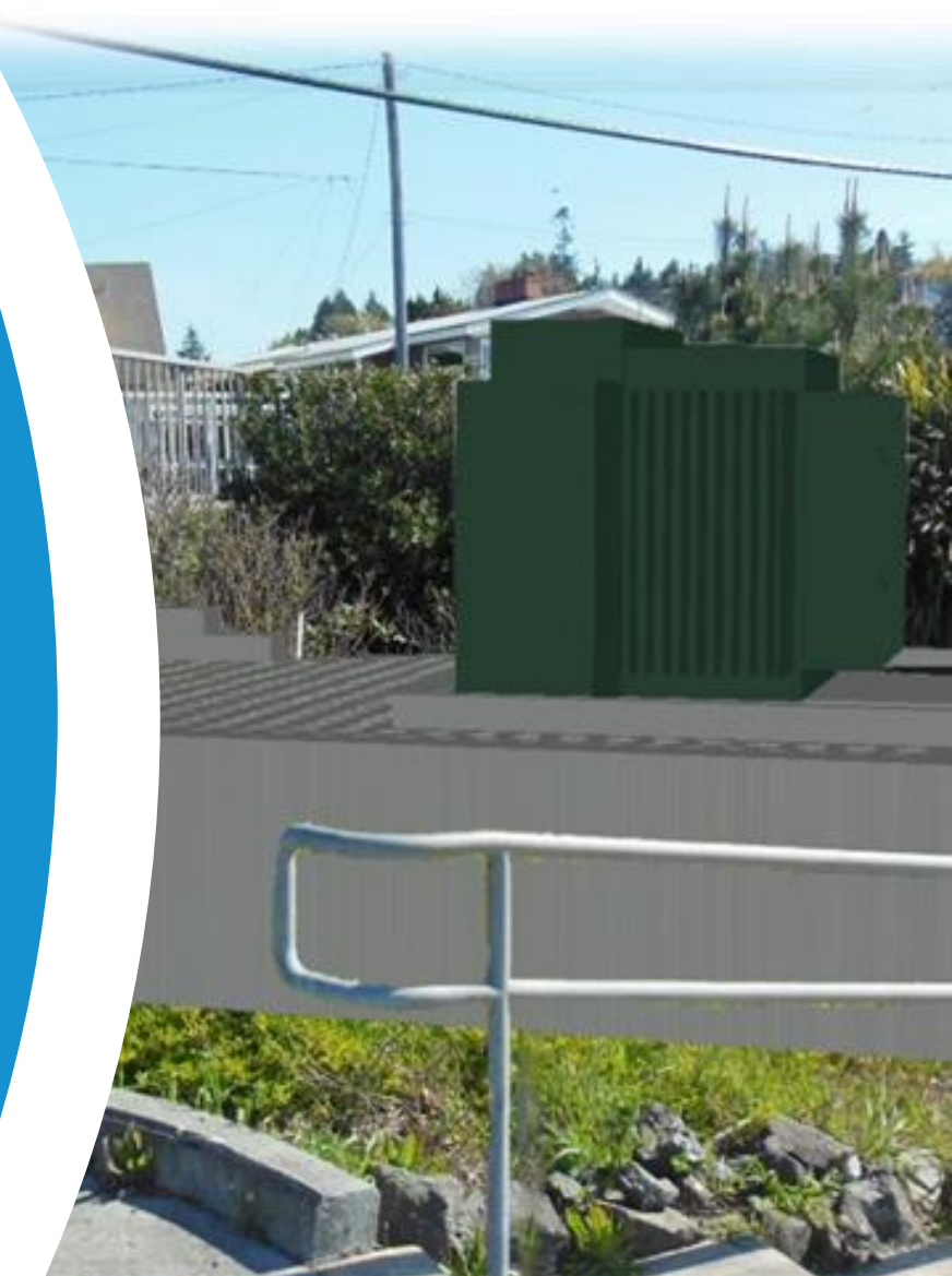
King County Alki Transformer
