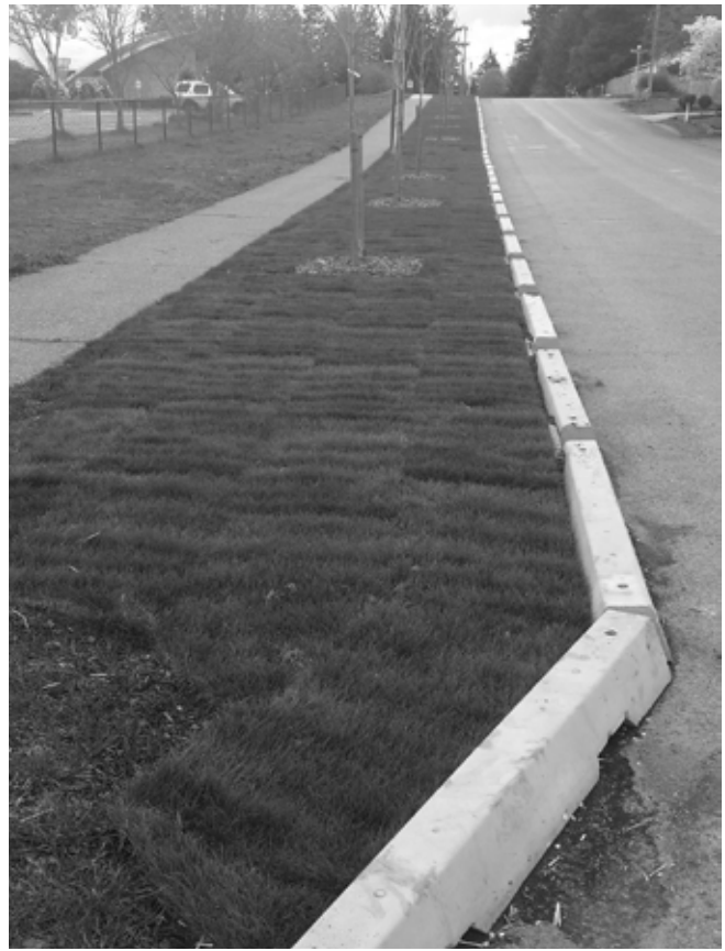
Low-cost improvements create safe spaces for pedestrians within the right-of-way and are nearly half the cost of traditional sidewalks. NE 135th Street is pictured above.
